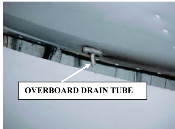
FIGURE 5 Fuel Pump Overboard Drain Tube (Typical)
